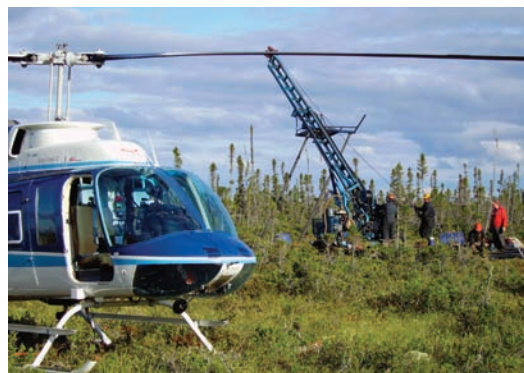
Diamond drilling at Probe's McFauld's Lake VMS prospect in the James Bay Lowlands of northern Ontario. Photo courtesy Probe Mines Ltd.
